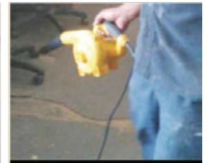
The construction site blows dust
